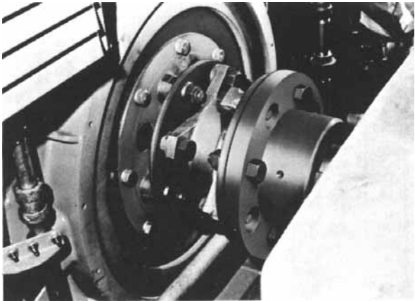
CMR coupling between engine and reciprocating compressor.
